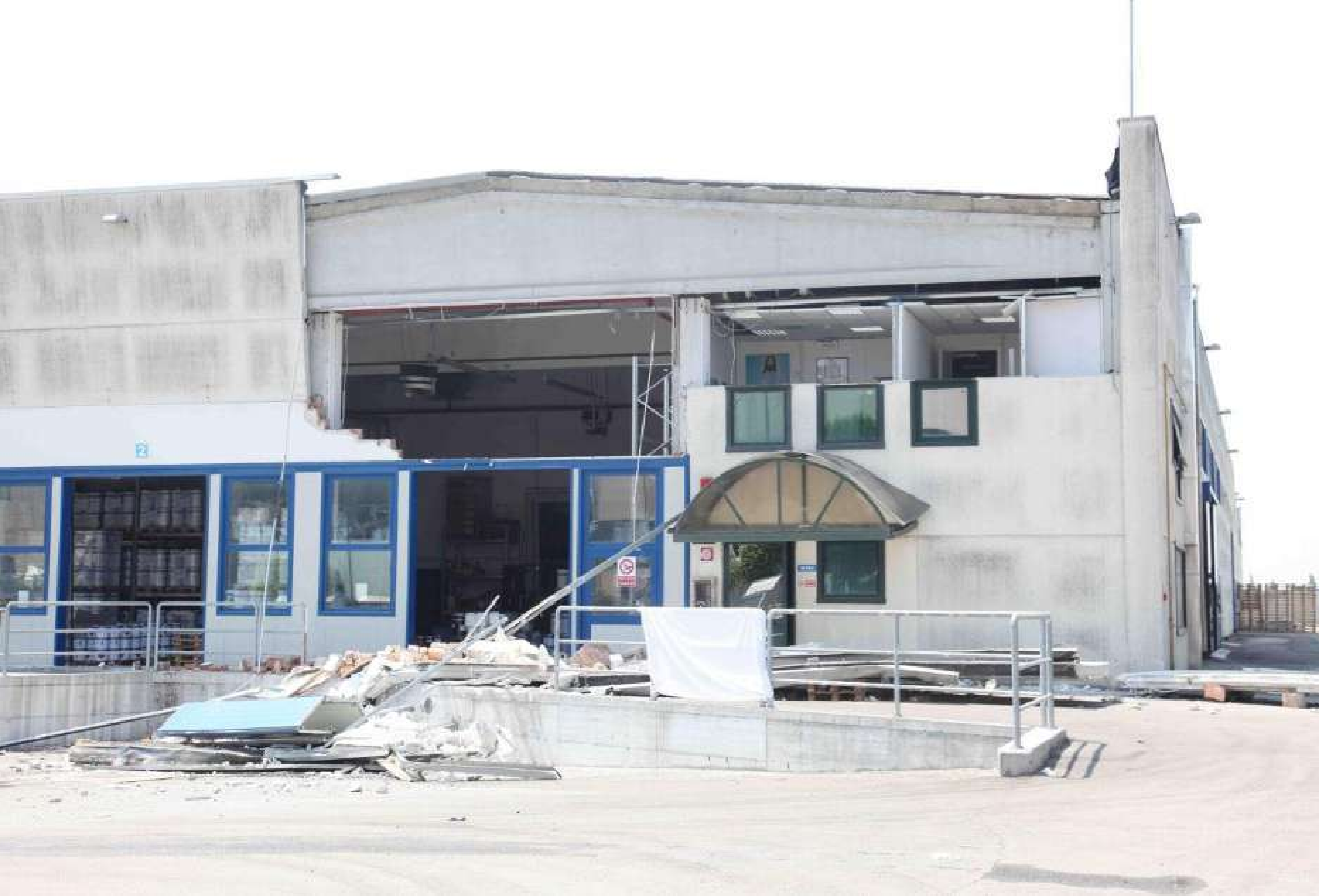
02. fanpage.it Danni e crolli nei capannoni prefabbricati durante il sisma del 2012 | fanpage.it Damage and collapses in the prefabricated warehouses during the 2012 earthquake
