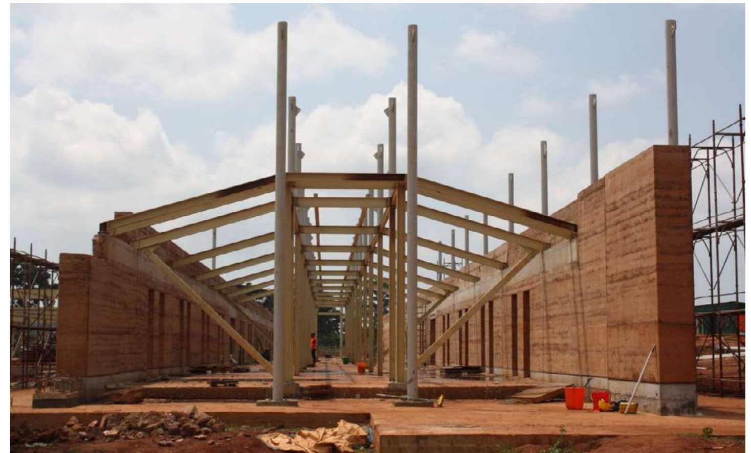
02. Vista padiglione di degenza in fase di cantiere | View of the hospital pavilion under construction. Photo and copyright: Emergency Archive
